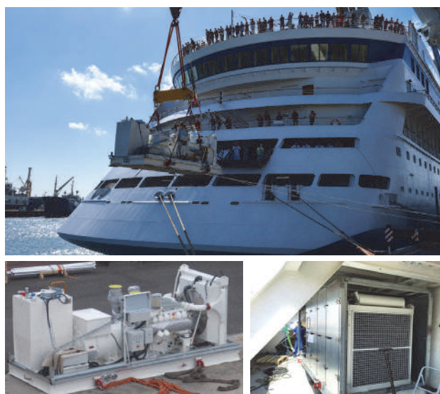
575 kWe Essential Genset with customised soundproof machine housing, installed on deck during a scheduled port call for uninterrupted cruise operation in a space limited engine room
